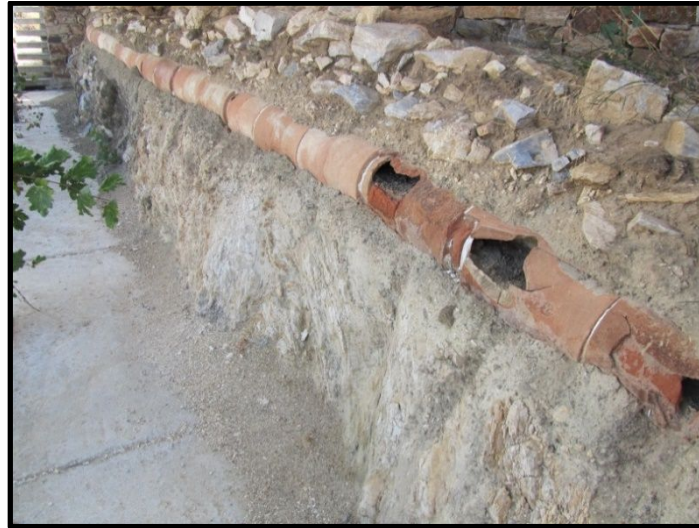
Picture 1. earth pipe has made earth
